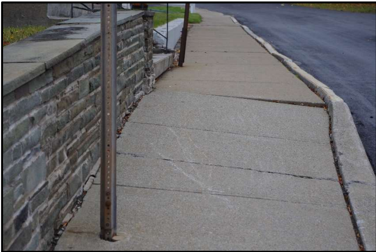
2020 – Existing sidewalk condition in Village
